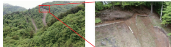
A distant view of a collapsed area (Photo taken by a drone)
