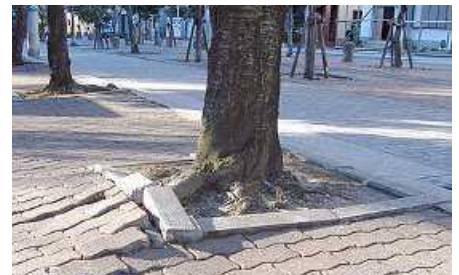
Uneven sidewalk due to rising tree roots
